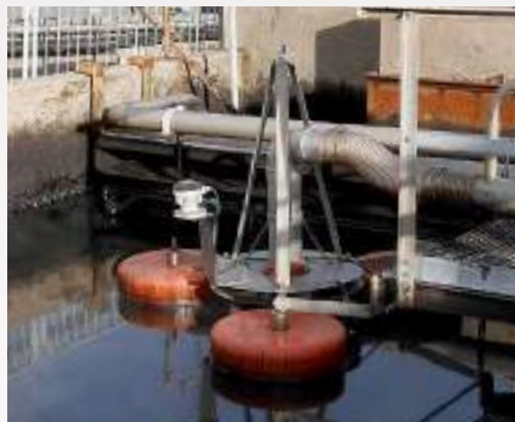
An Ultra-SurfCleaner operating in an API separator.
